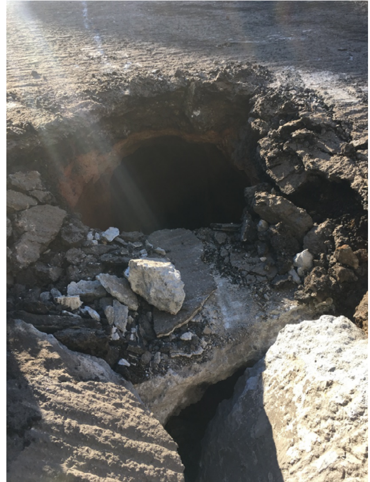
Sinkhole found on Sunset Avenue
