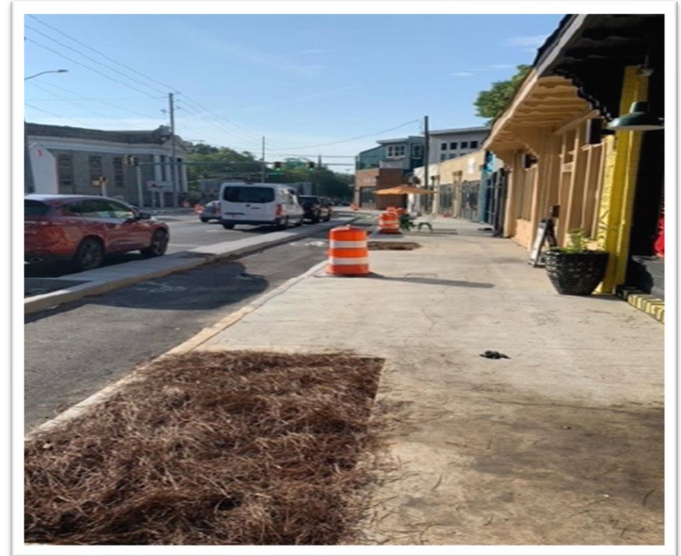
New sidewalks and protected bike lane installed on Ralph David Abernathy Boulevard
