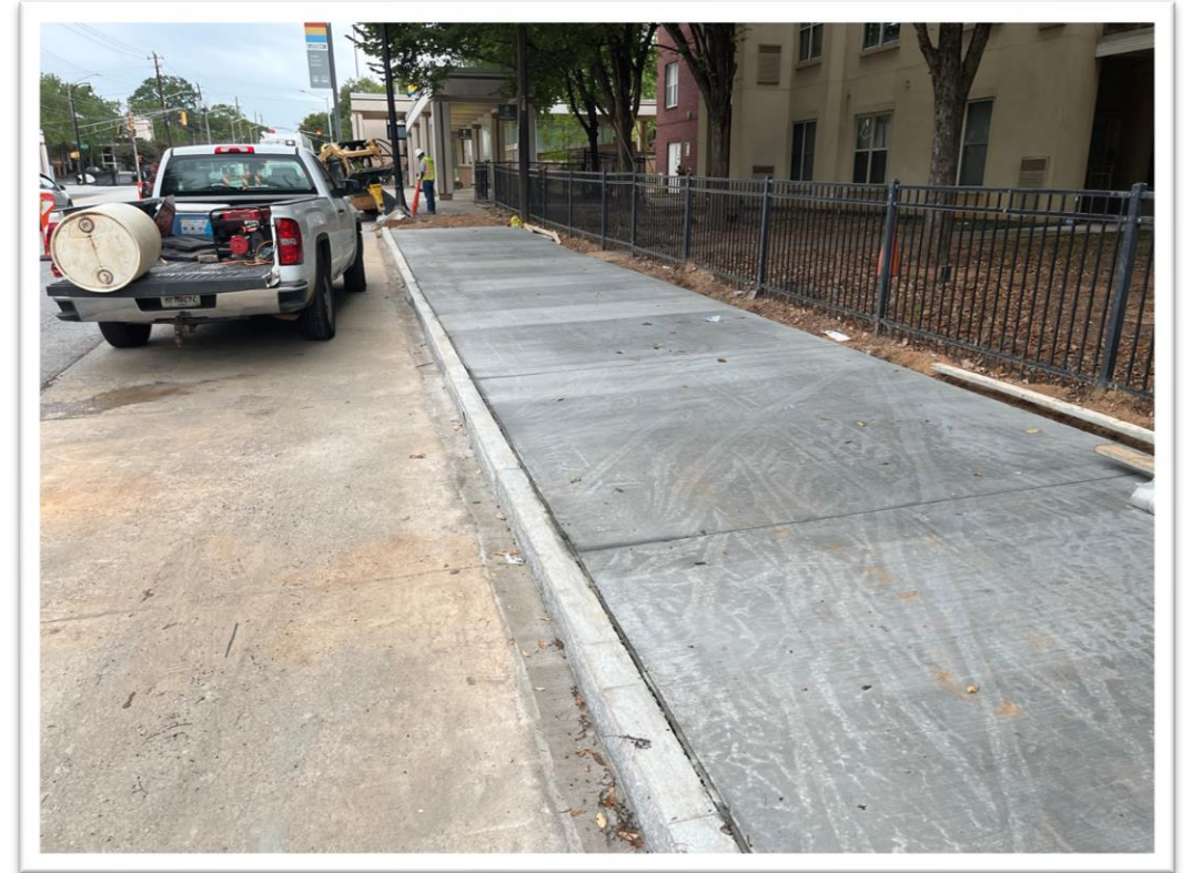
New sidewalk poured along Joseph E. Lowery Boulevard as part of the complete street project
