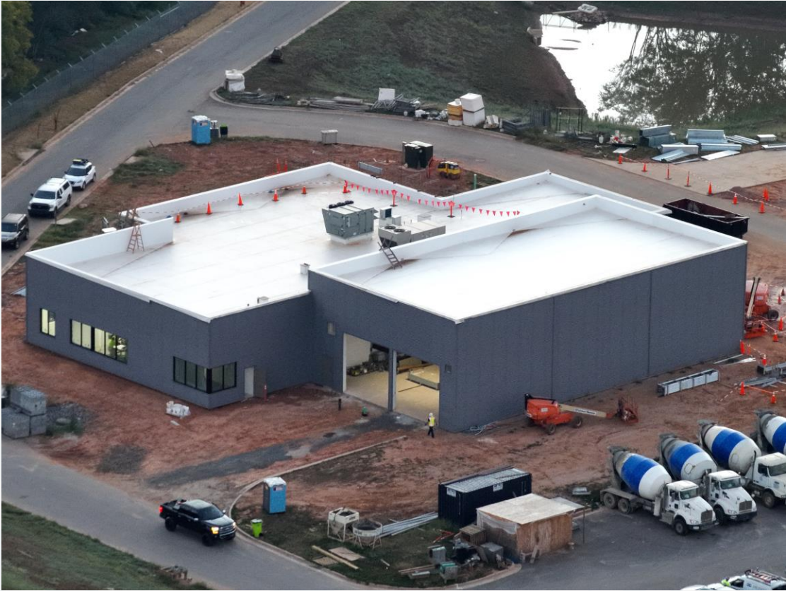
Training Fire Station
