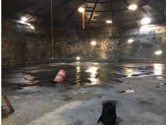
Centrate Storage Tank
