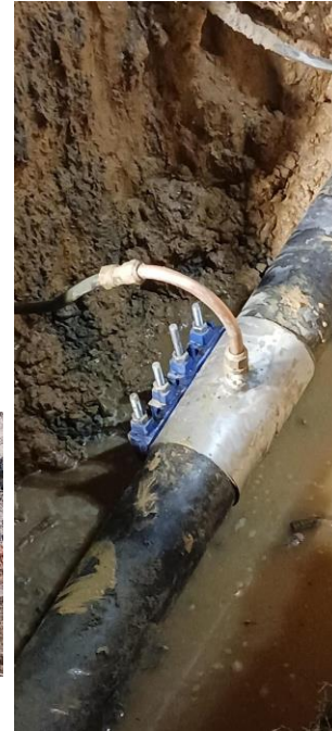
Service Line Leak
