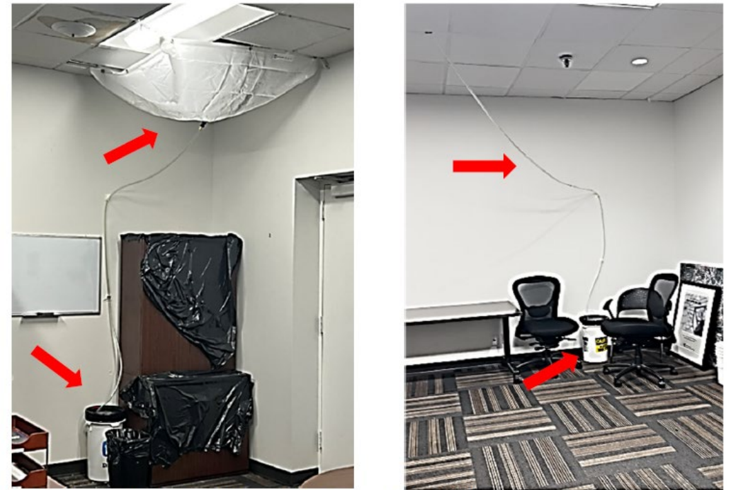
Exhibit 3: Police Precinct Sustained Water Damage After Renovations
