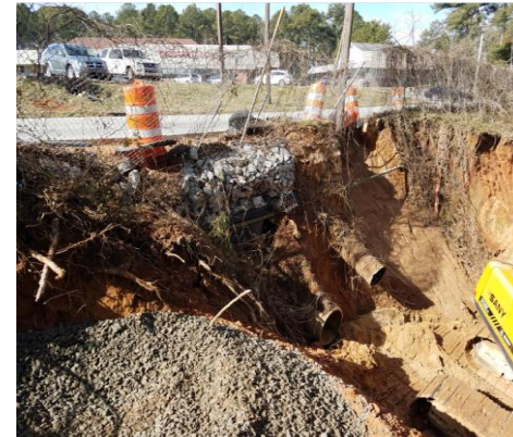
2275 Mt. Gilead Road SW Embankment Washout
