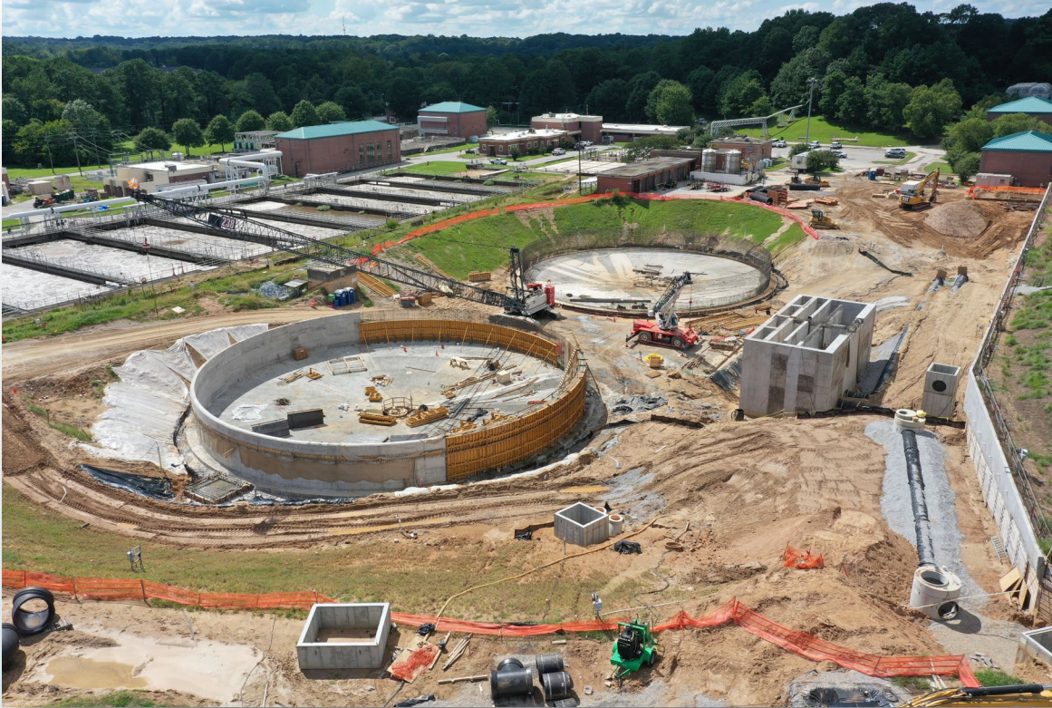
South River WRC showing new clarifiers
