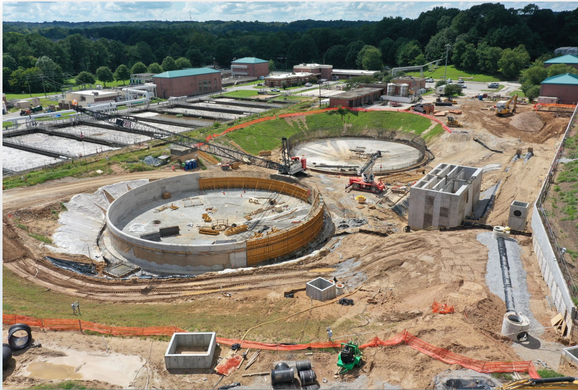
South River WRC showing new clarifiers
