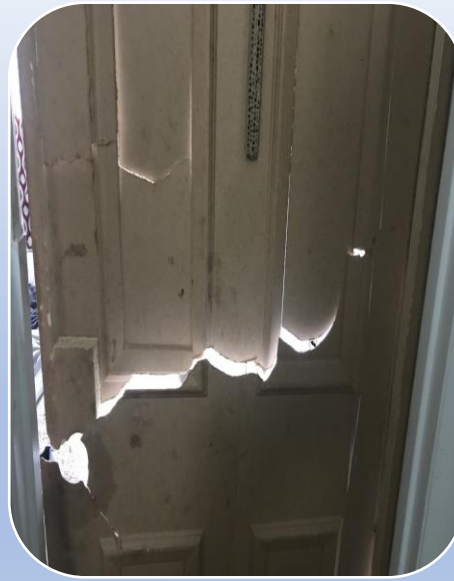
Damaged bedroom door
