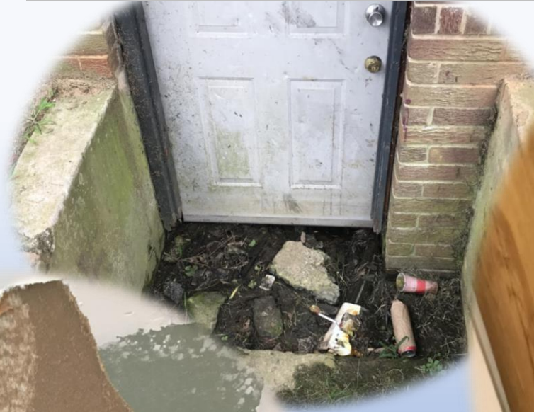
Standing water at basement door
