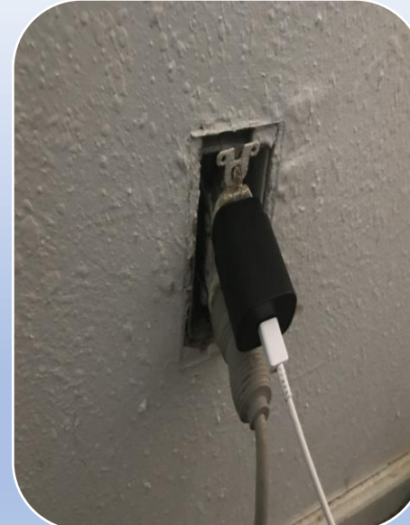
Missing cover plates
