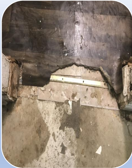
Interior floor damage - kitchen
