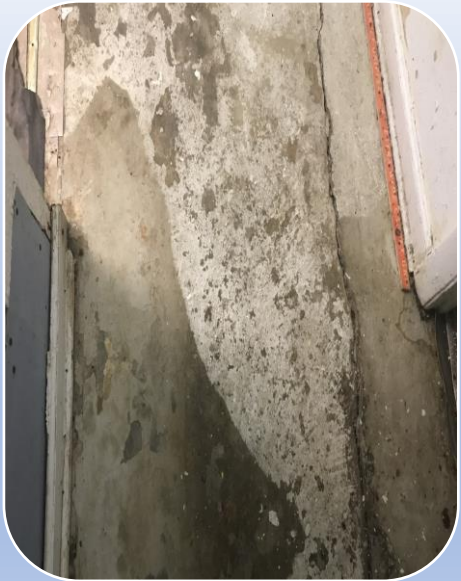
Interior floor damage - hallway
